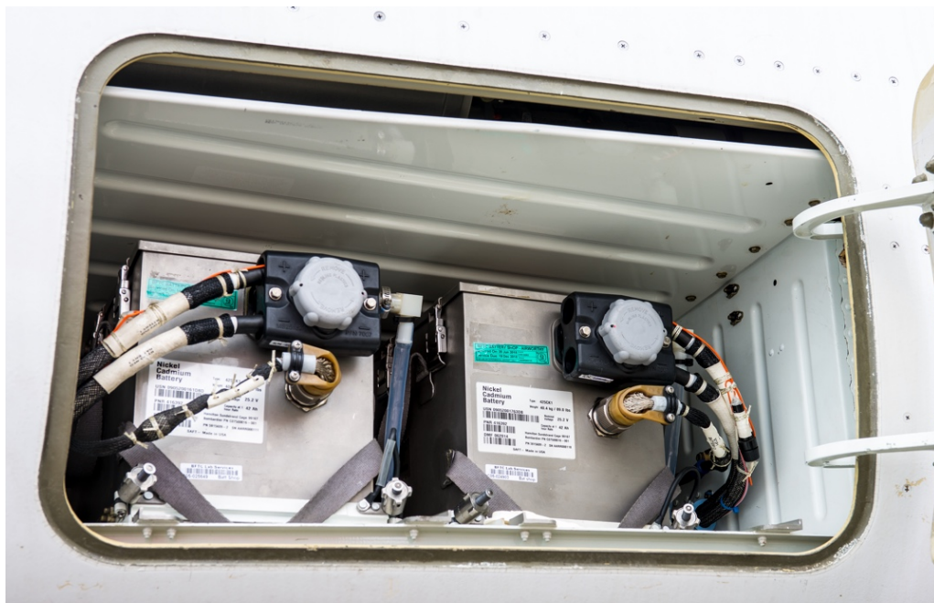
Figure 2.1. : compartiment des batteries (photo © Pierre Gillard).
